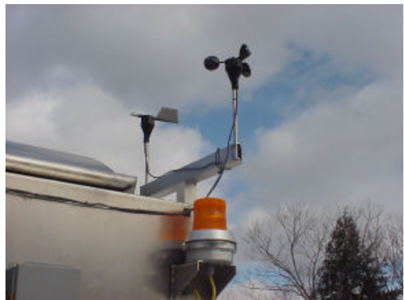
Anemometer and wind vane mounted on roof of MERV provides surface wind speed and direction.
